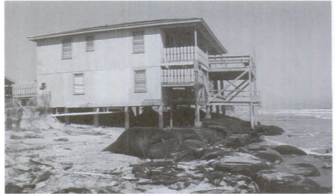
Michigan, Pennsylvania, New Jersey, North Carolina, and South Carolina were eligible to certify structures in danger of imminent collapse, under the Upton-Jones provisions of the NFIP.
