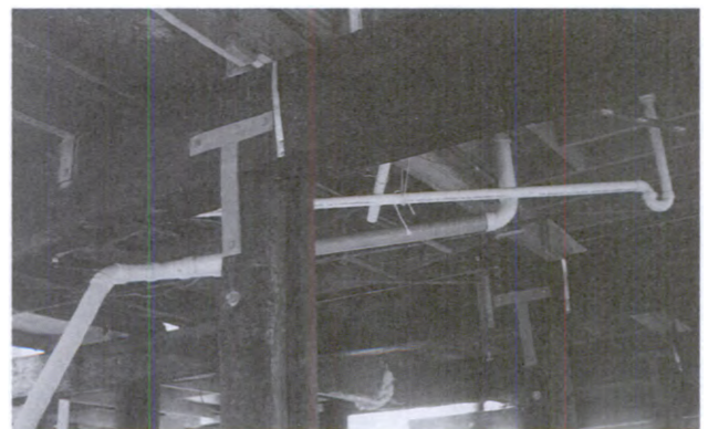
The cross beams supporting the structure rest on one pile and are bolted into the second pile with a steel T-strap.
