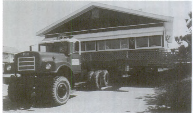
Relocation involves separating the building from its existing foundation and transporting it to a new location, where it is placed on a new foundation.
