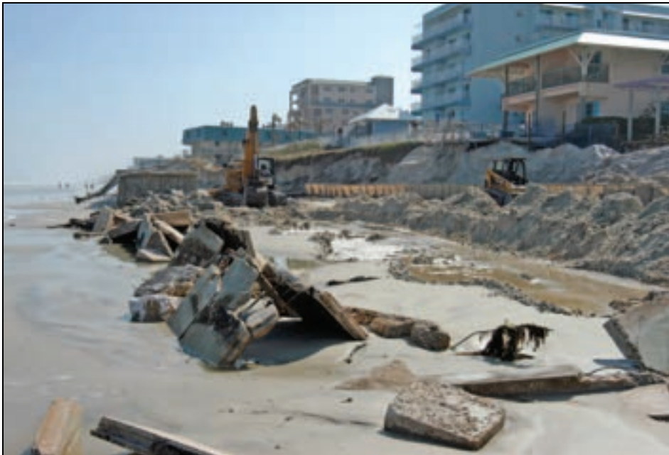
Figure 3-32. Erosion and seawall damage in New Smyrna Beach, FL, following Hurricane Jeanne in 2007
