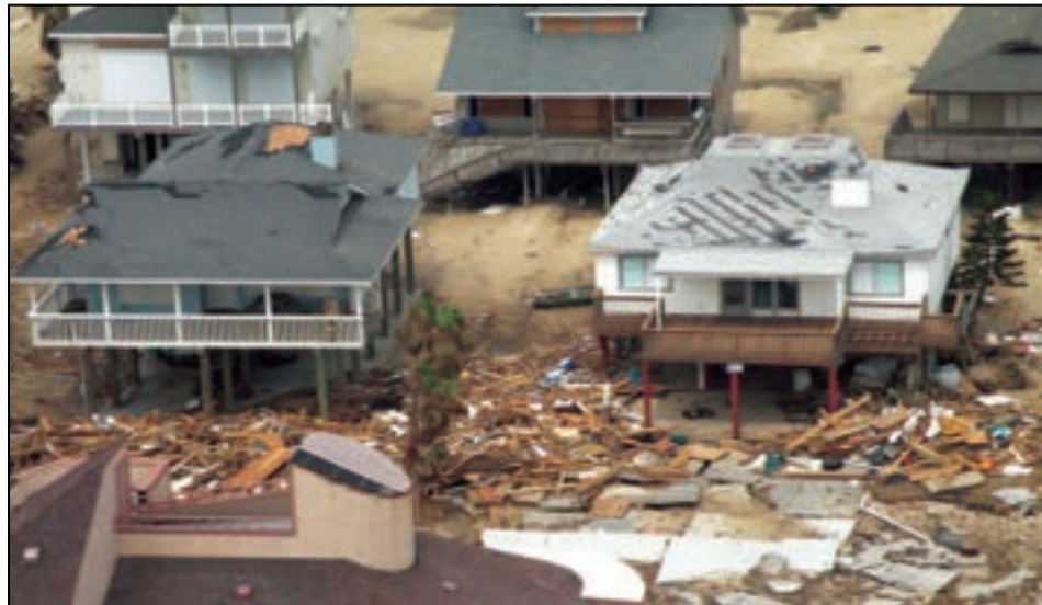
Figure 2-11. Galveston Island beach house with wind damage to roof in high pressure zones at roof edge and roof corners, Hurricane Ike, 2008
