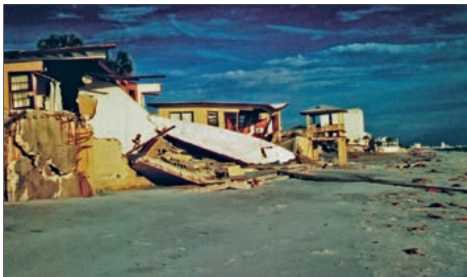
Figure 3-45. Failure of seawall in Bay County, FL, led to undermining and collapse of the building behind the wall (Hurricane Opal, 1995)
