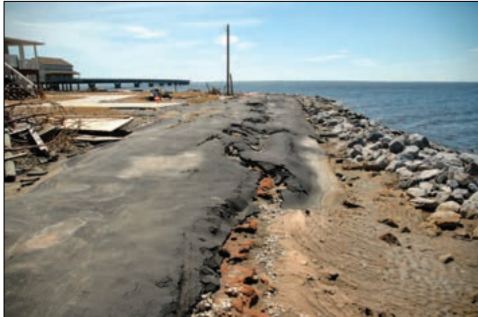
Figure 4-11. Roads placed near shorelines can wash out, causing access problems for homes such as these located at Garcon Point, FL (Hurricane Ivan, 2004)
