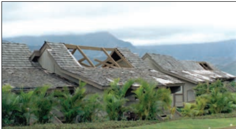
Figure 3-9. Loss of roof sheathing due to improper nailing design and schedule in Kauai County, HI (Hurricane Iniki, 1992)
