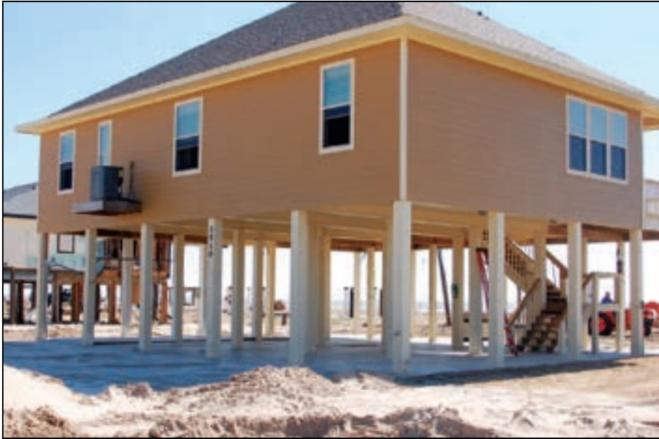
Figure 2-19. Breakaway walls below the first floor of this house broke as intended under the flood forces of Hurricane Ike (Bolivar Peninsula, TX, 2008)
