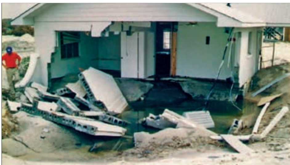
Figure 2-13. Extreme case of localized scour undermining a Zone A continuous perimeter wall foundation located several hundred feet from the shoreline, Hurricane Fran (Topsail Island, NC, 1996)
