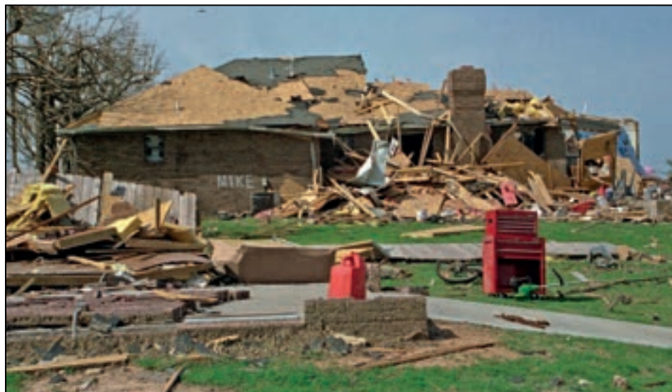
Figure 2-4. Roof structure failure due to inadequate bracing and inadequate fastening of the roof deck, Hurricane Andrew (Dade County, FL, 1992)
