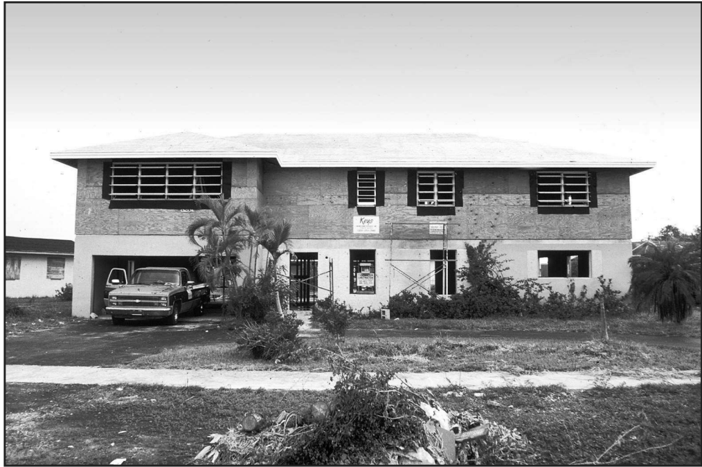
Figure 62 After the wood framing was completed, the roof and exterior wall sheathing were added.
