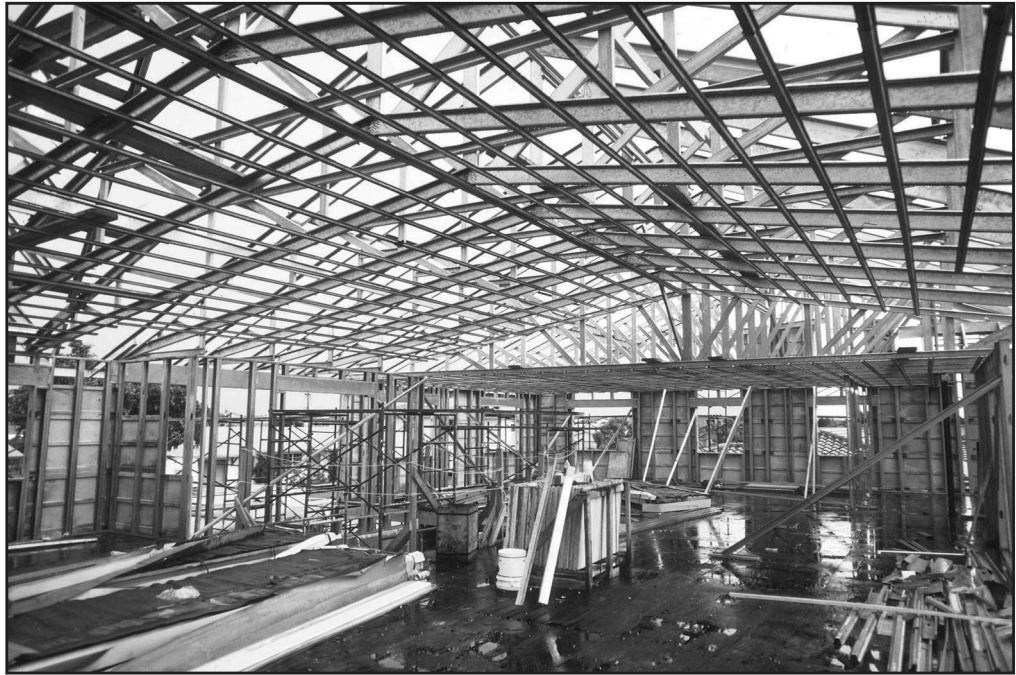
Figure 54 Metal framing is used for the new second story, including the walls and roof support system.
