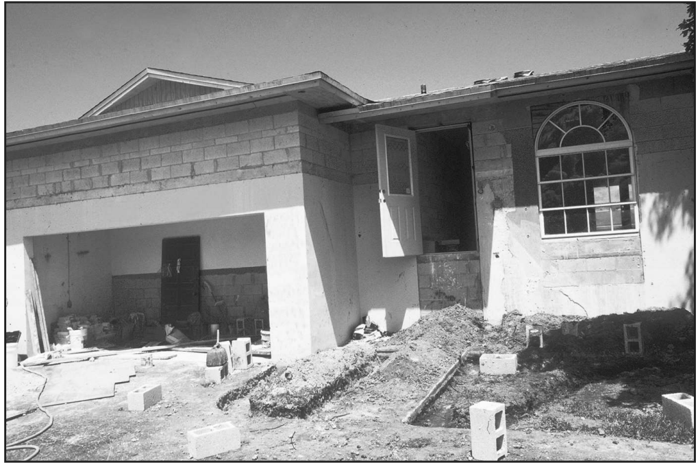
Figure 29 Windows and doors are added. The height of the raised front door shows the amount of elevation.
